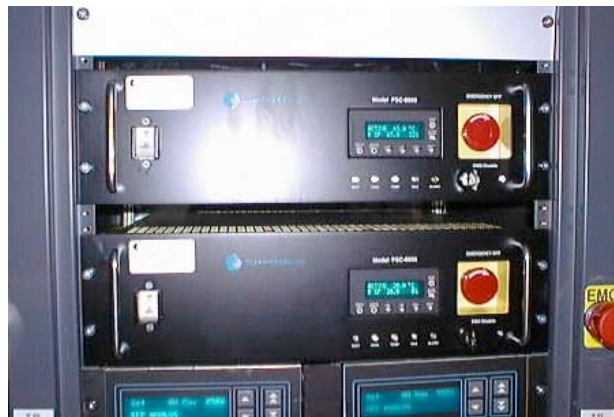
Figure 5. PSCs installed in tool's rack
