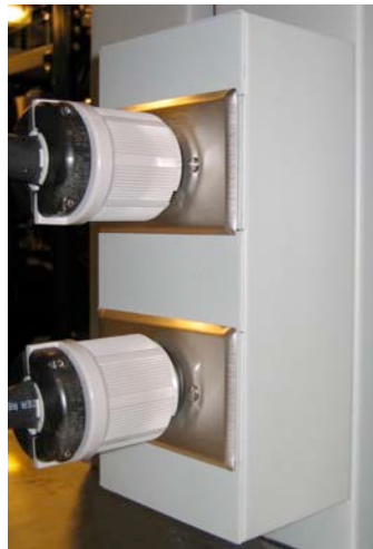
Figure 9. Facility-supplied Power Receptacles
